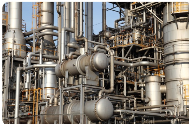
Figure 4 -This oil refinery processes crude oil into usable energy sources, such as gasoline.
